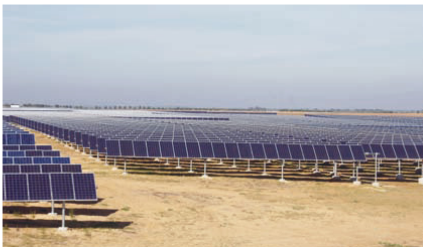
Figura 4.6 – Planta Solar Fotovoltaica de 10 MWp, on grid (IEA/PVSP, 2009)
